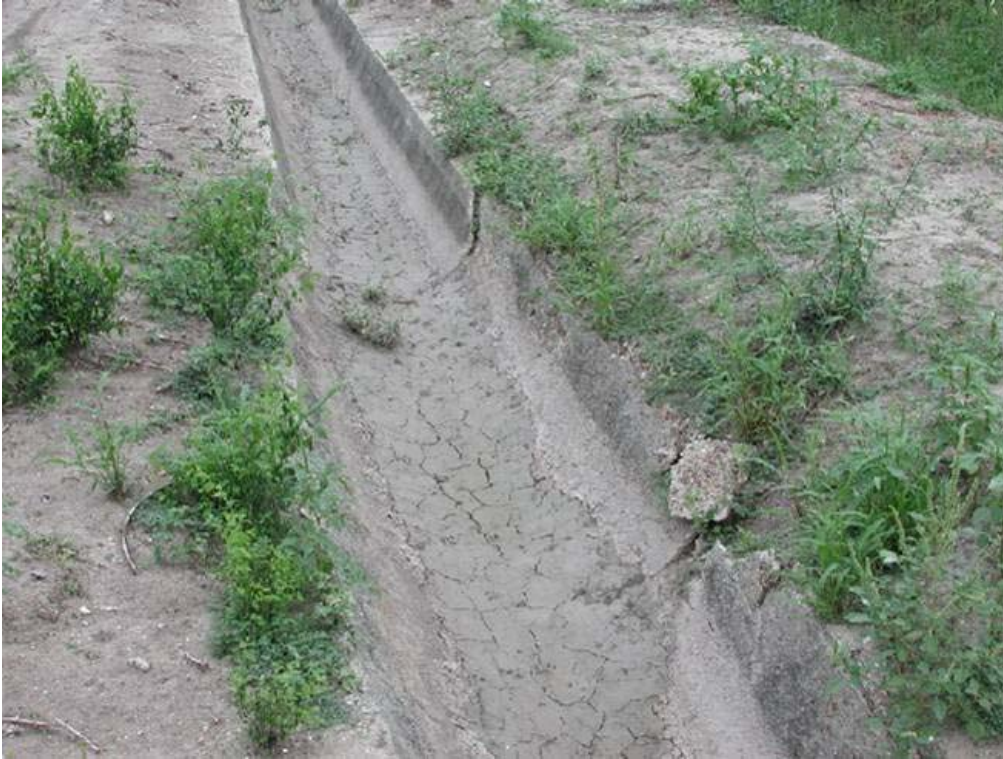
Figure 3. Example of large cracks (D), 5 to 10 feet apart.
