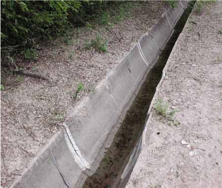
Figure 6. This canal has severe shifting of side walls, with pencil-size cracks (C) less than 5 feet apart.
