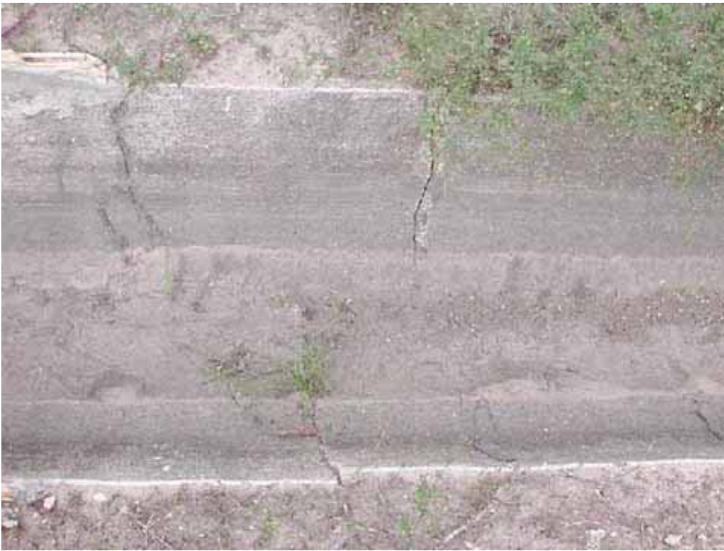
Figure 7. This photograph shows hair-line cracks (B), less than 3 feet apart.
