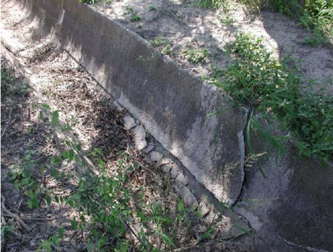
Figure 8. This canal has major damage to the right side wall and a large crack (D) which will eventually result in the wall falling into the canal.
