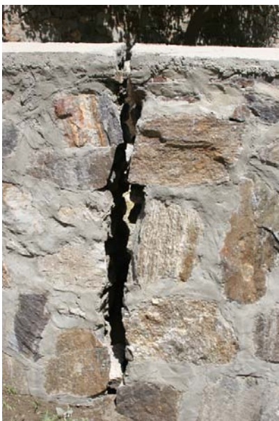
Expanding crack in same retaining wall
