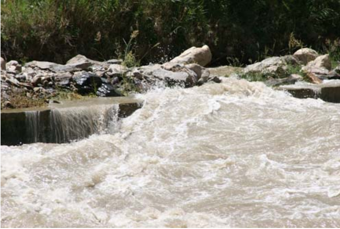
Hydraulic jump and water washing over retaining walls put the structure in jeopardy
