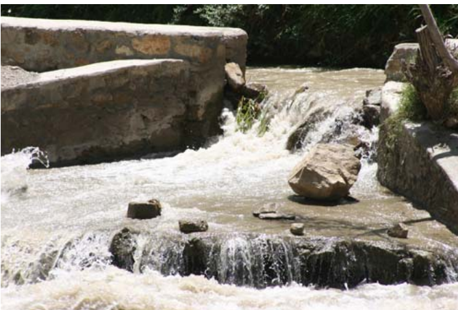
Erosion of spillway and retaining walls, questionable use of rock and mortar construction at this critical location
