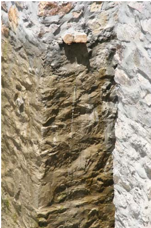
Water leaking through structure
