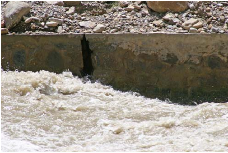
Large crack in retaining wall, evidence of likely structure failure in the next few years
