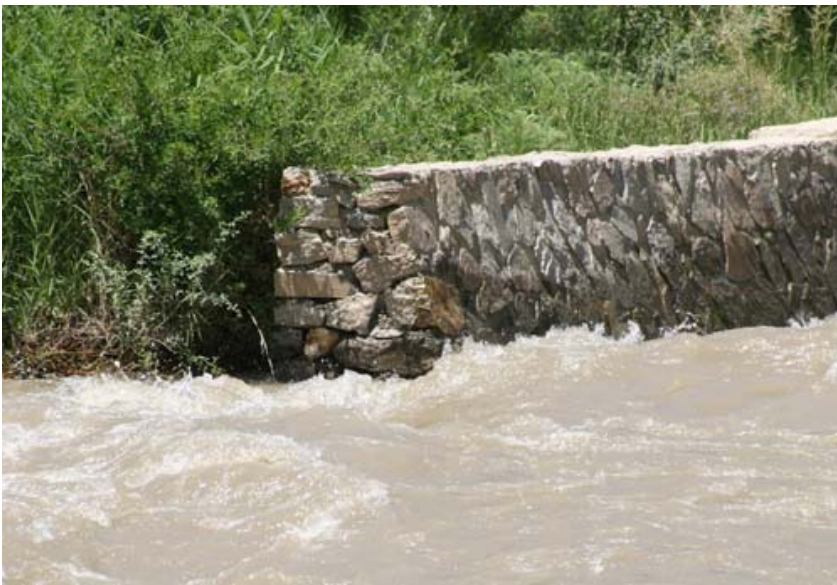
Eroding rock and mortar construction
