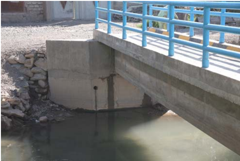
Bridge/aqueduct combination – two large leaking cracks at the base of the aqueduct are undermining structural integrity
