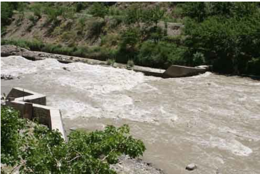
Improper design of structure: inadequate or no accommodation of the hydraulic jump
