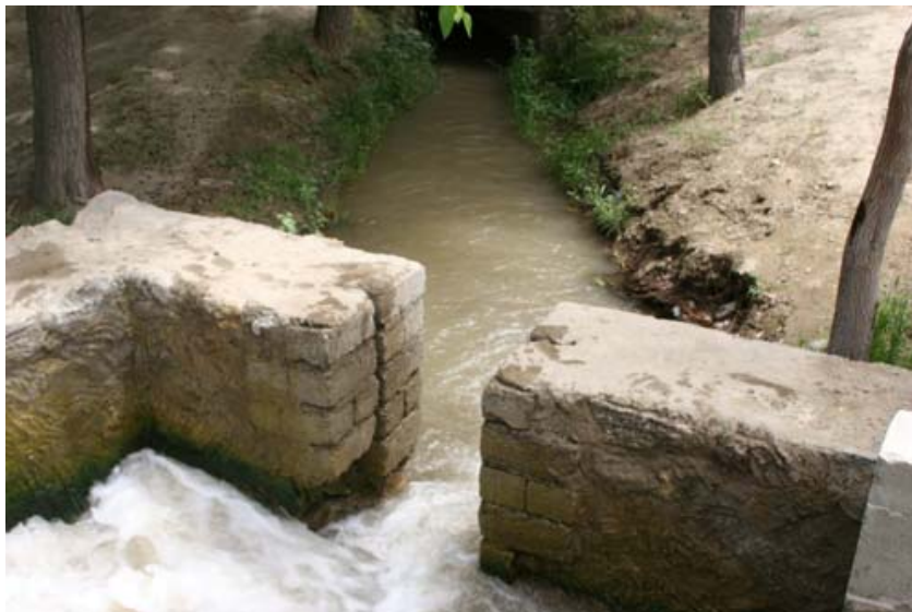
Erosion of structure at critical location
