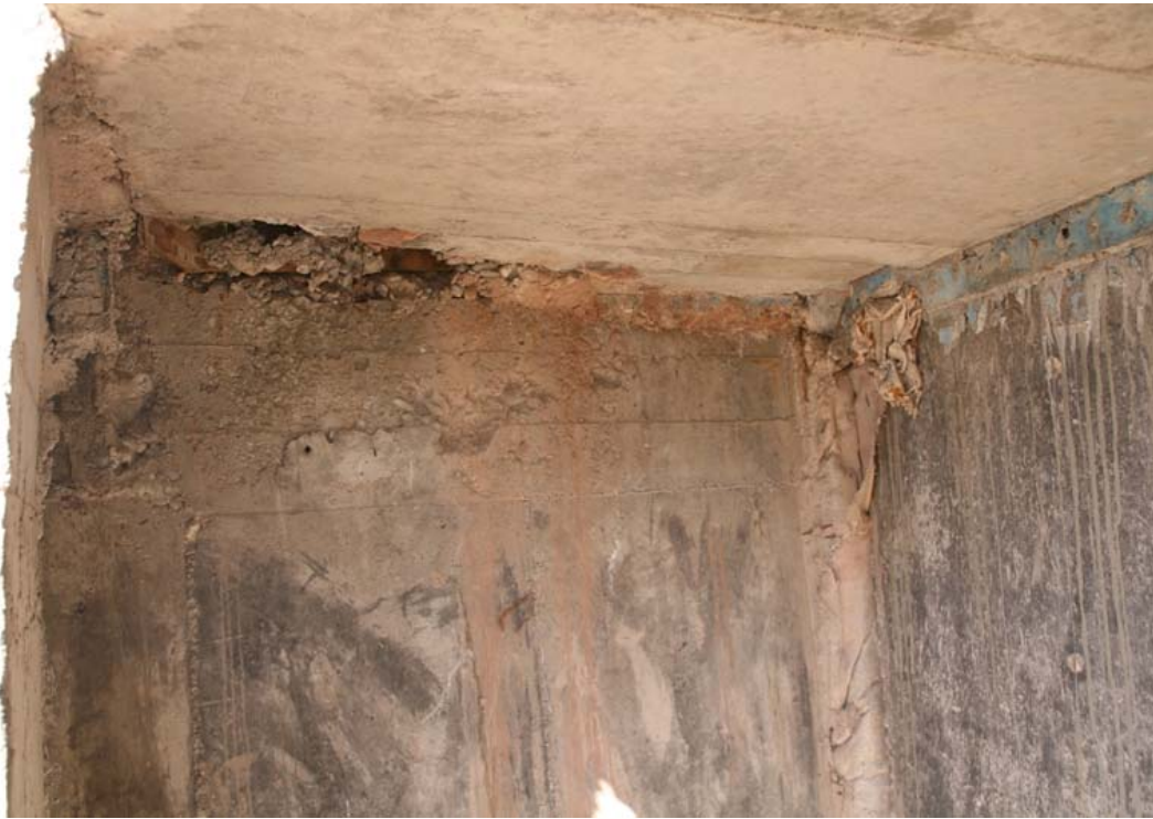
Poor workmanship and quality control – creates weak spots at a critical area in structure
