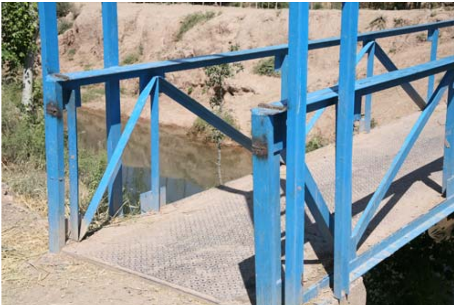
Sloppy and rusting welds
